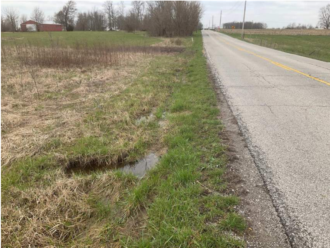
3. Looking W at maintained roadside on the south side of East 281 st Street.
