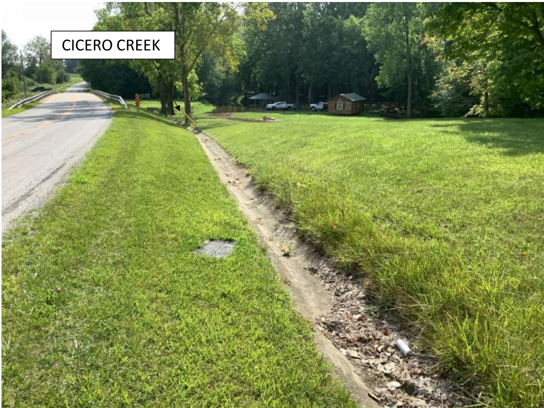
34. Facing southeast looking at RSD 5 and maintained roadside. Cicero Creek in the background. Photo taken 08/08/2023.
