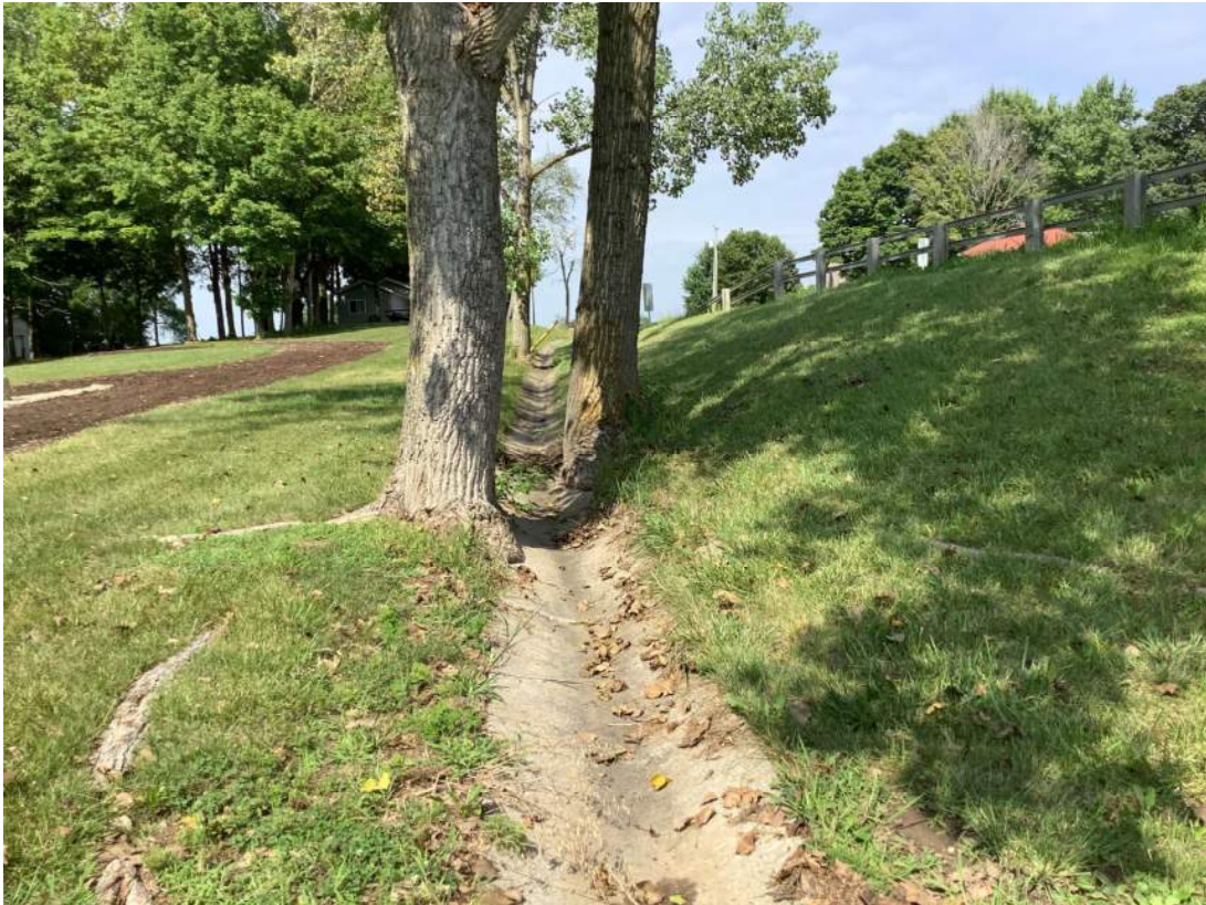
37. Facing west just south of 281 st St. looking at RSD 5. Photo taken 08/08/2023.
