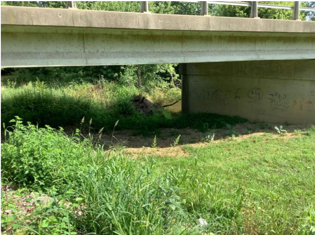
38. Facing north just south of 281 st St. looking at Structure 29-00064 which carries 281 st St. over Cicero Creek. Photo taken 08/08/2023.
