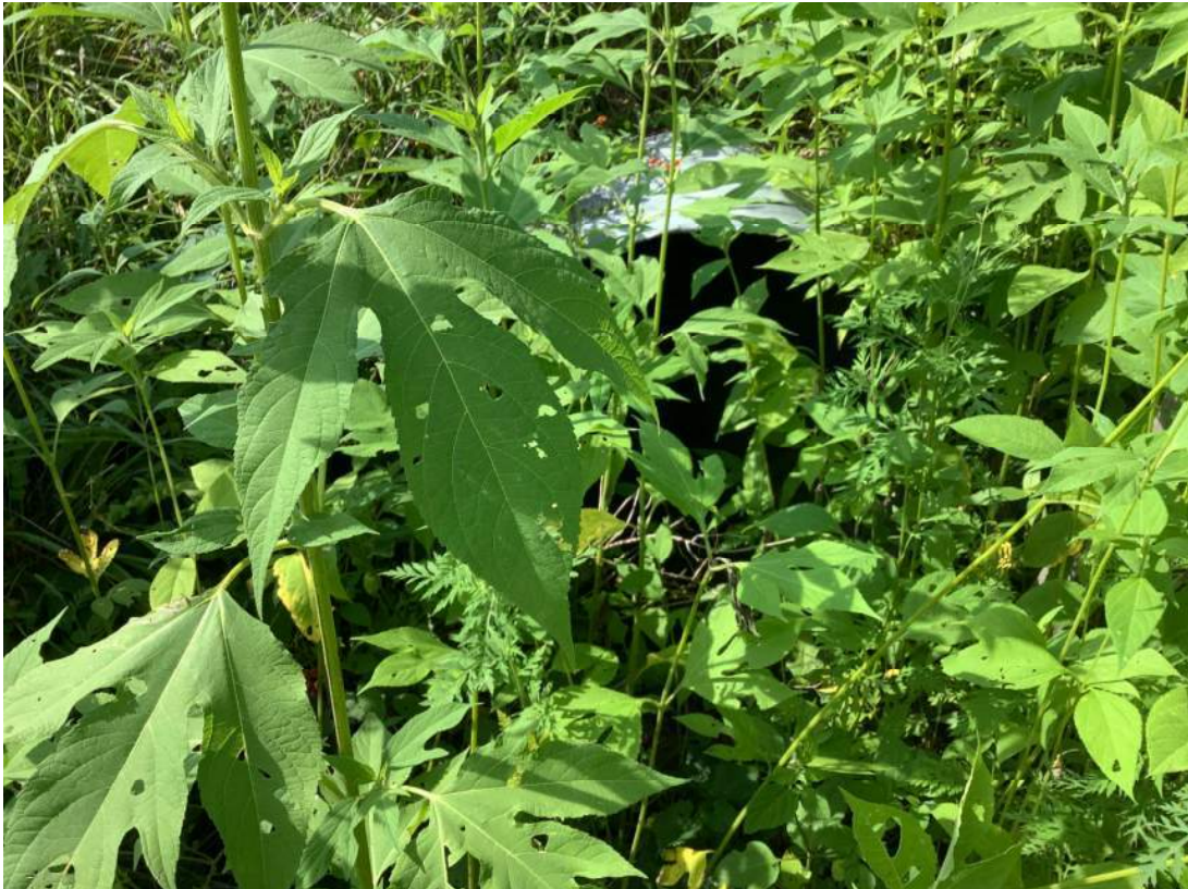
22. Facing south just north of 281 st St. looking at inlet of structure. Photo taken 08/08/2023. .
