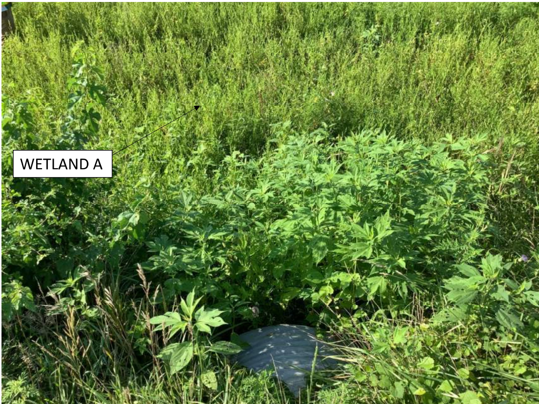
6. Facing south just south of 281 st St looking at outlet of structure and Wetland A in the background. Photo taken 08/08/2023.
