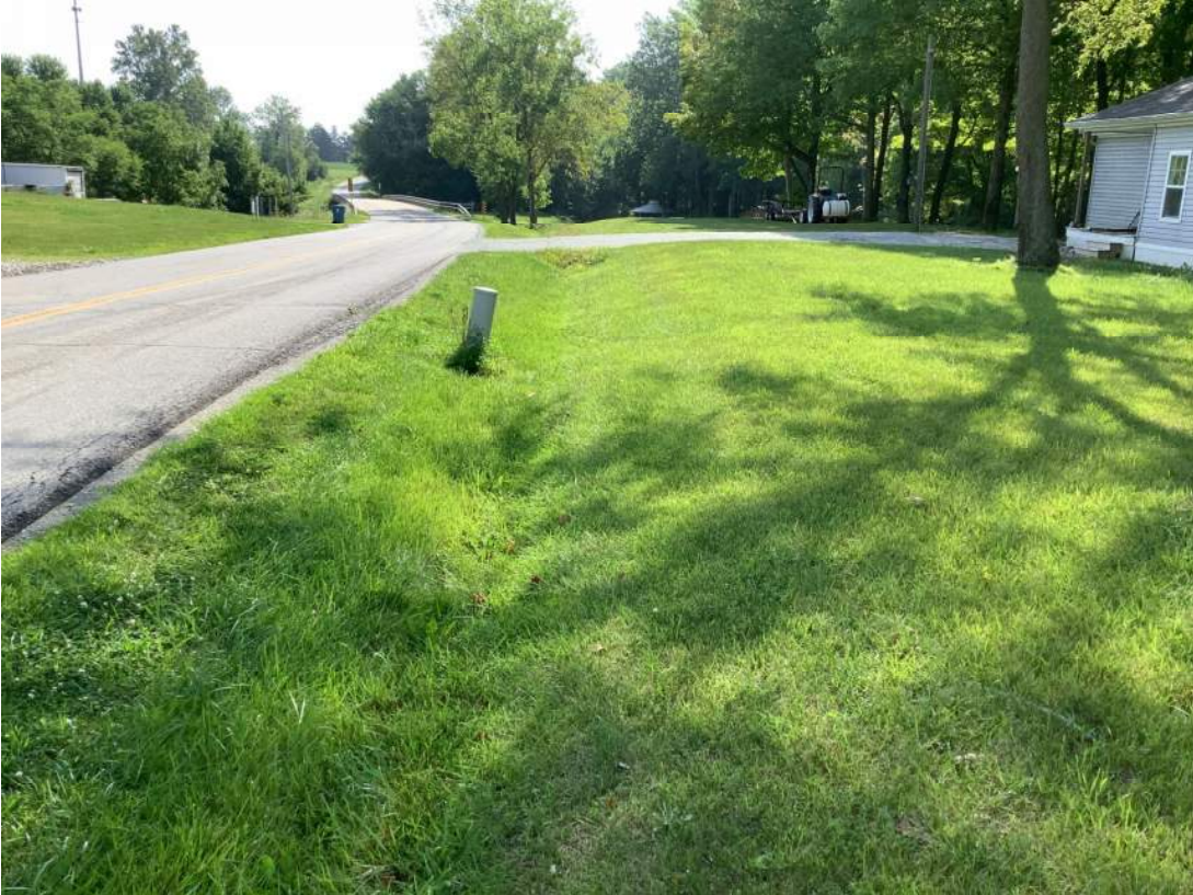
31. Facing east just south of 281 st St. looking at RSD 3 and maintained roadside. Photo taken 08/08/2023.
