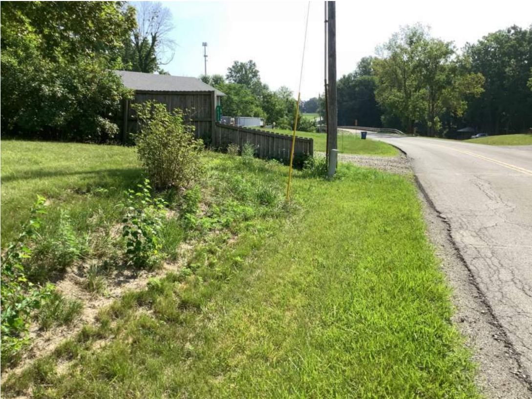
32. Facing east just north of 281 st St. looking at RDS 4 and maintained roadside. Photo taken 08/08/2023.
