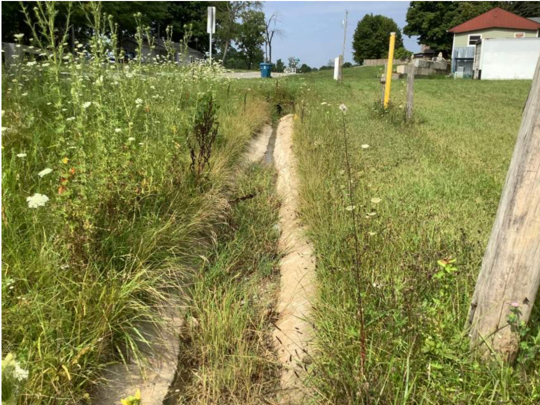
39. Facing west just north of 281 st St. looking at RSD 6 and roadside. Photo taken 08/08/2023.
