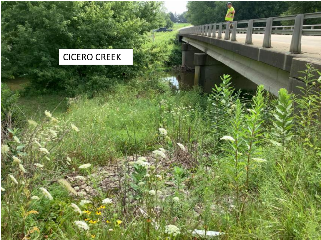
40. Facing east looking at Little Cicero Creek under structure NBI: 400046. Photo taken 08/08/2023.
