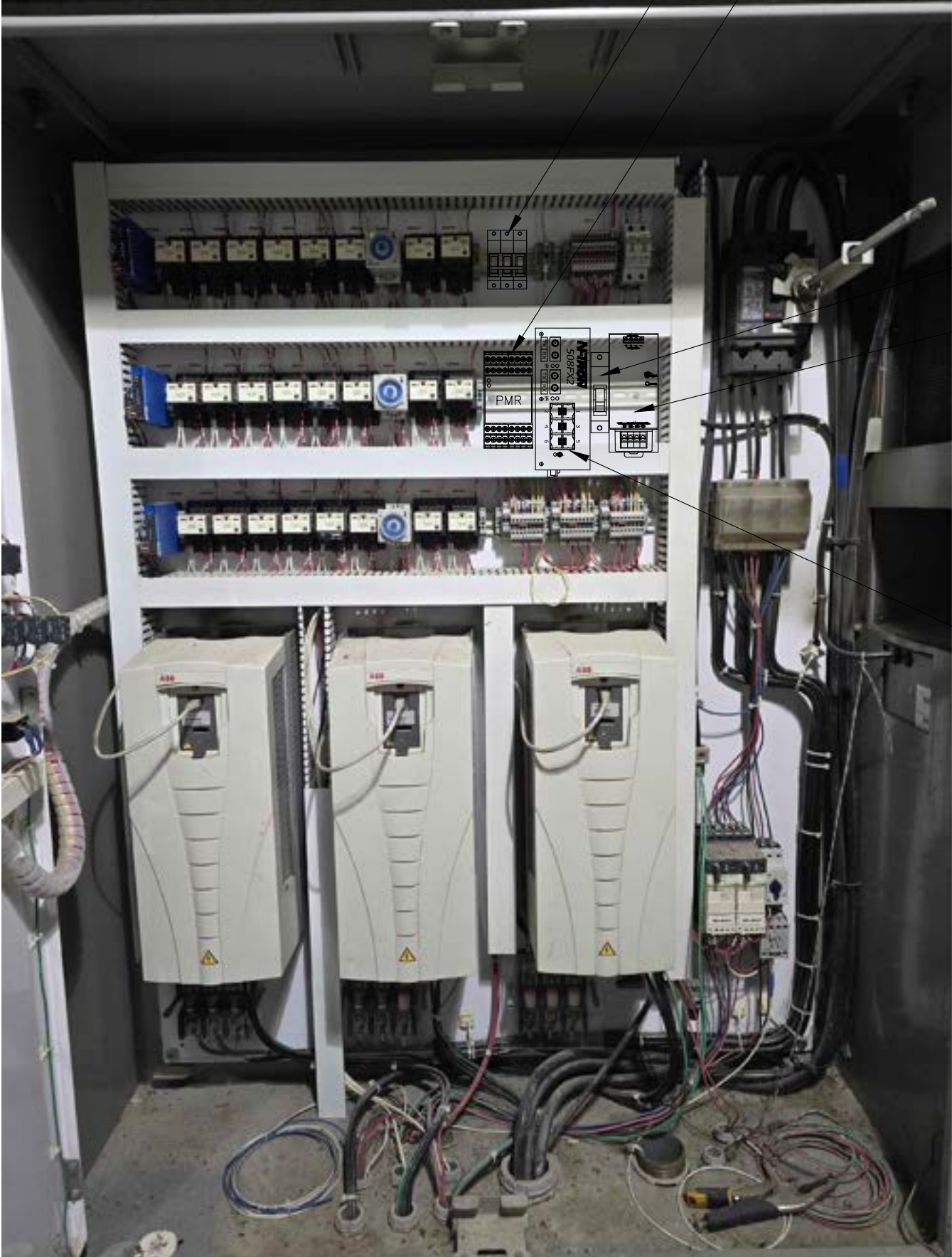
TRIPLEX BLOWER CONTROL PANEL EQUIPMENT PANEL
