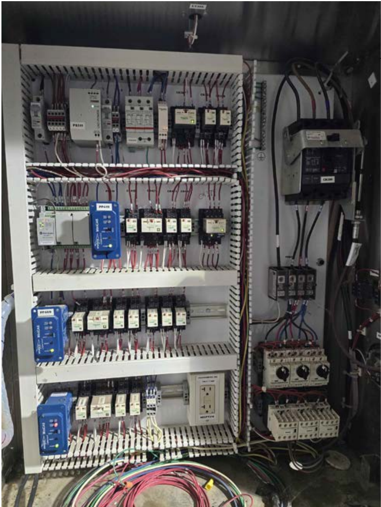
RAS/WAS EQUIPMENT PANEL
