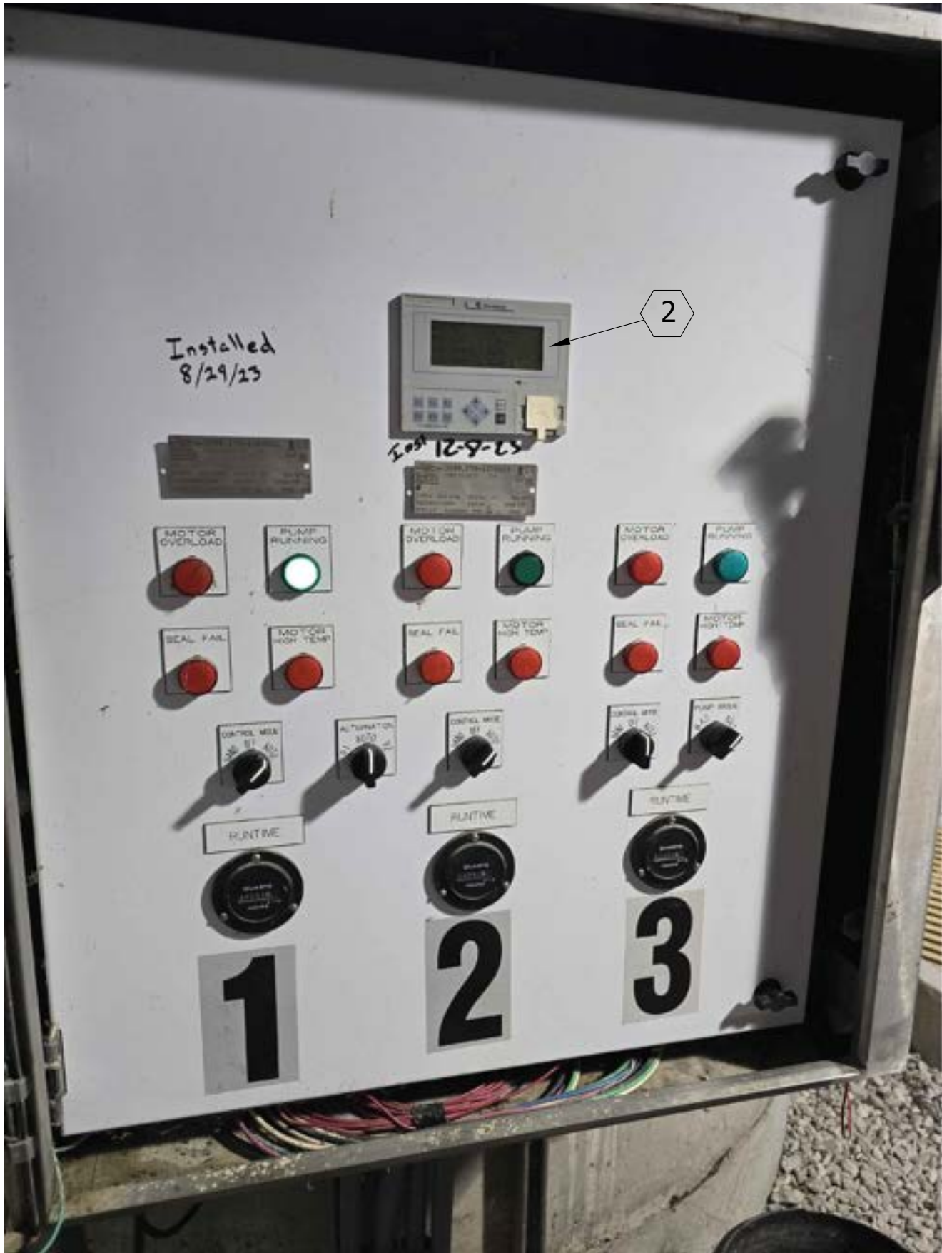
RAS/WAS SWING OUT PANEL
